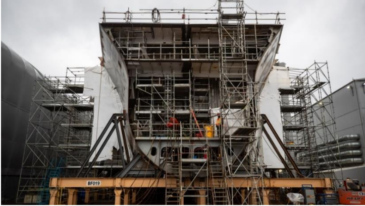
A worker stands on a Joint Support Ship being built for the Royal Canadian Navy at Seaspan Shipyards in North Vancouver, BC,
