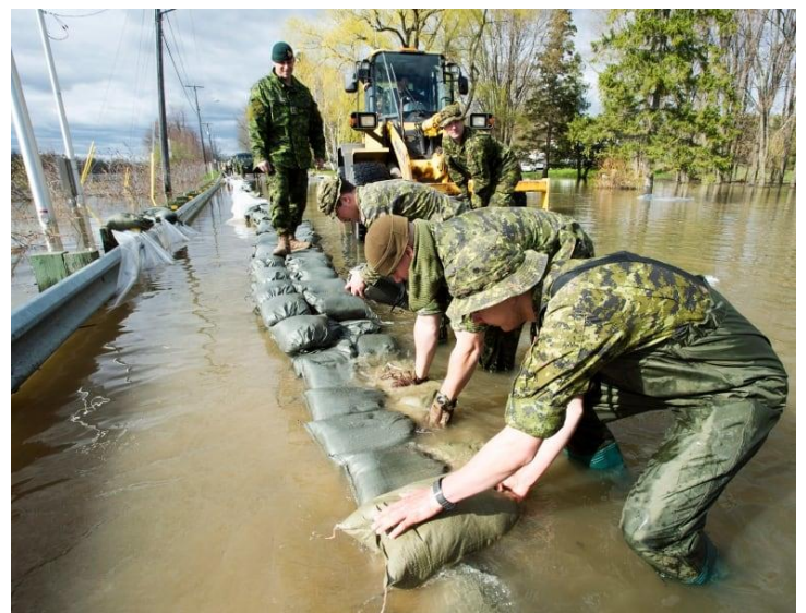
Canadian Forces members can be deployed almost anywhere and need gear that holds up to a variety of environments from the battlefield to flood zones. In this photo, soldiers place sandbags to reinforce the highway in Saint-Andre-d'Argenteuil, Que., after flooding in the area in 2017. (Ryan Remiorz/Canadian Press)
