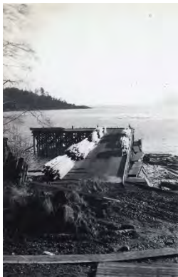
2C – Dock Area. The dock floorboards have been completed and there is a quantity of rebar ready to be used on the next concrete job. The Officers’ Quarters foundation is being worked on. 15FdMuseum989.154.55
